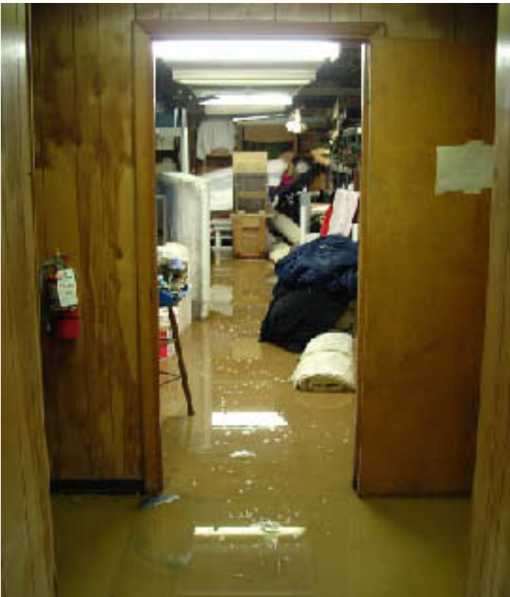
Overhead lights reflect in the muddy water standing in the basement’s center room.
